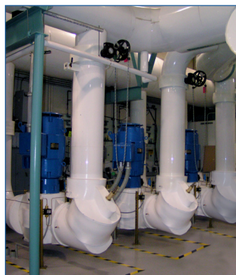
District Cooling Project, Phoenix, U.S.A.
